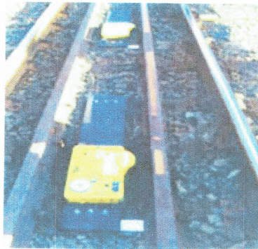
Example of a pair of Balises between guard rails. Note the cable connected to the 'controlled' balise in the background
