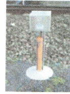
Trackside Junction Box
