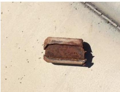
Broken hinge pin support
